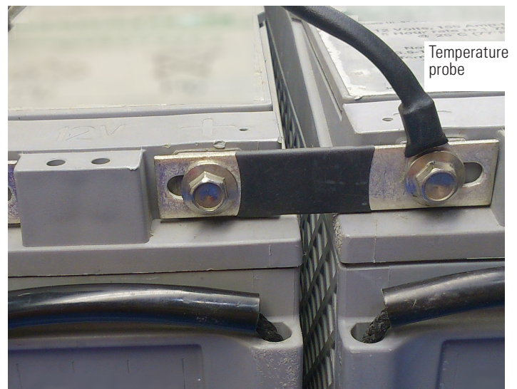
Figure 48: Battery temperature probes, battery bay
