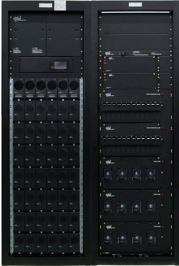
CXPS-C Plant with (8) x 4.6kW rectifier shelves (48 modules) next to a distribution bay
