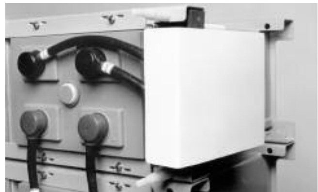
Figure 9: Outer shield attached to the main terminal take-offs
