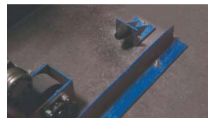
Gantry Crane guide rail
