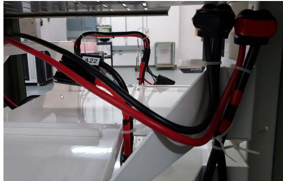
Fig. 4-15, Tying THHN/THWN Heavy Gauge Battery Cables
